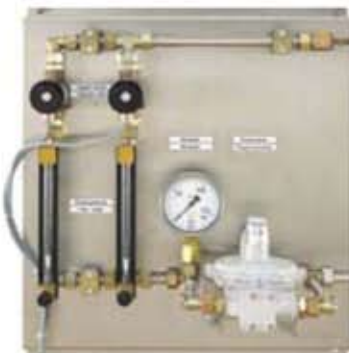
10. Automatic N2 feed system
