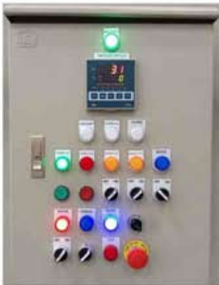
Digital Controller Panel burner
