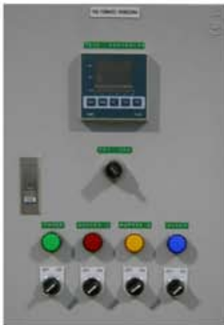
Digital Controller Panel burner
