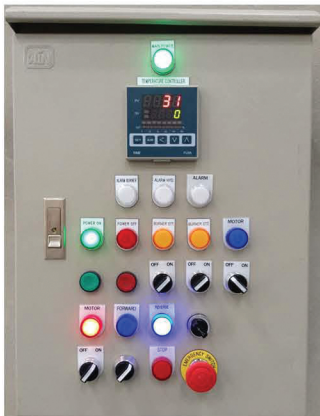
Digital Controller Panel burner
