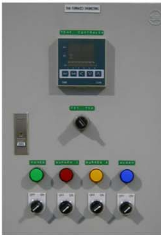
Digital Controller Panel burner
